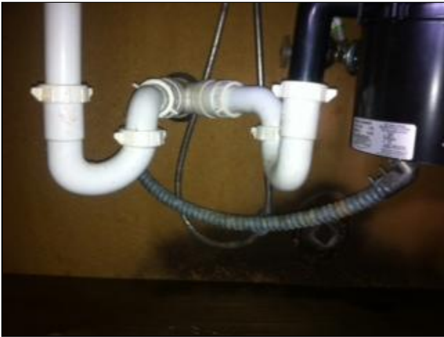
6.0 Picture 1 plumbing waste drain
