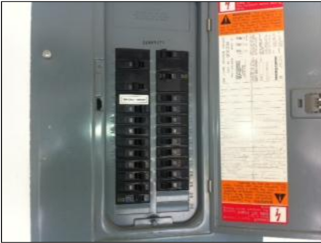
7.6 Picture 2 distribution panel
