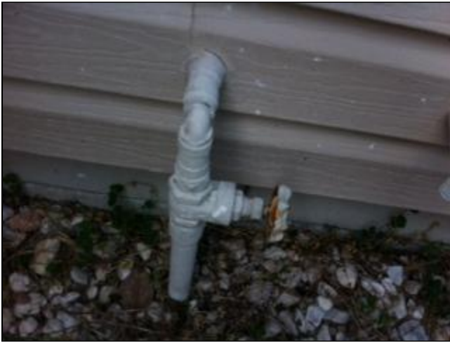
6.3 Picture 1 water shutoff
