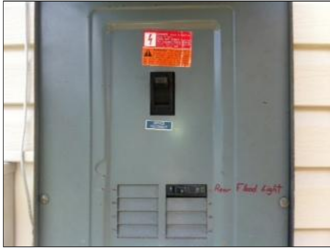
7.6 Picture 1 main panel
