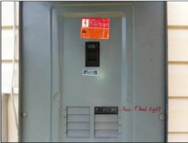
7.1 Picture 1 main panel
