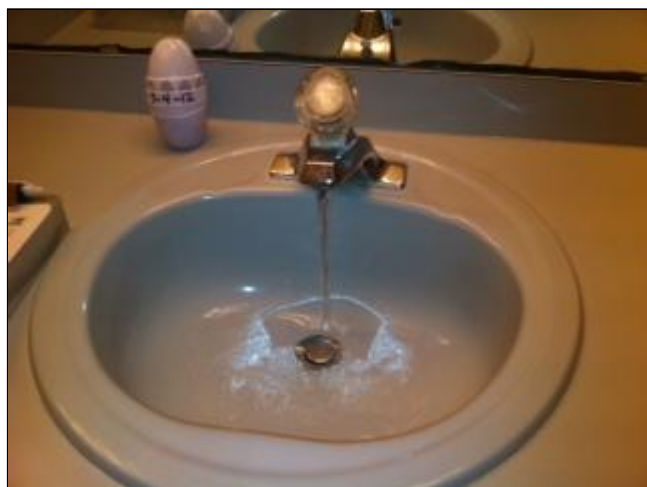
6.1 Picture 1 hot water distribution
