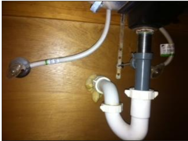
6.0 Picture 2 plumbing waste drain
