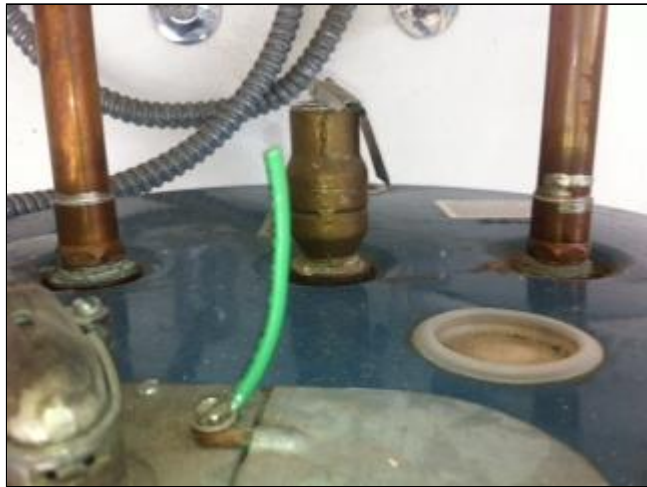
6.2 Picture 2 TPR valve
