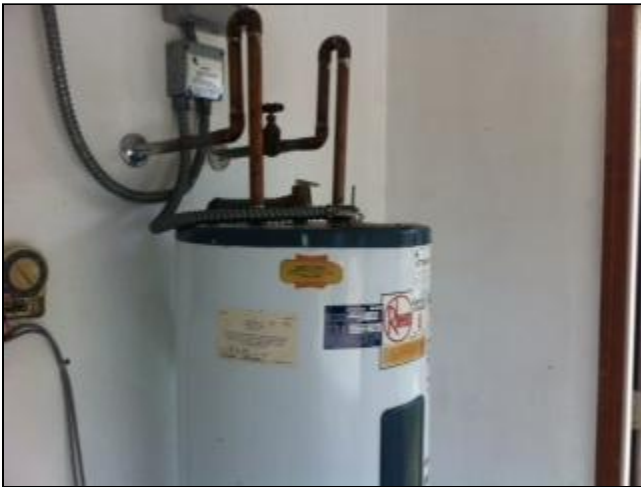
6.2 Picture 1 water heater
