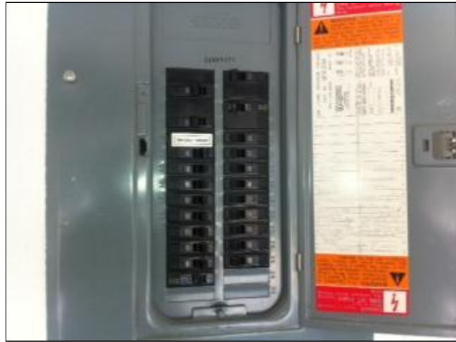
7.1 Picture 2 distribution panel
