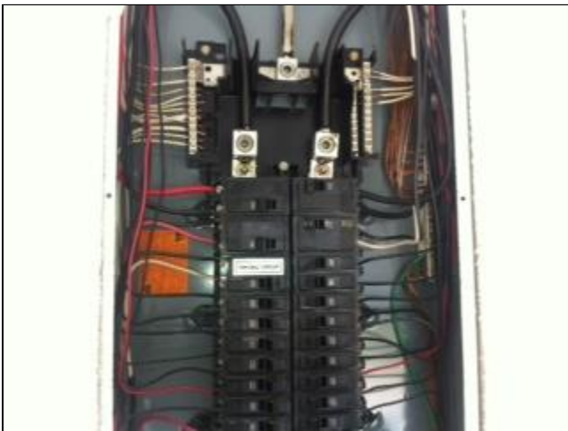
7.1 Picture 3 overcurrent protection
