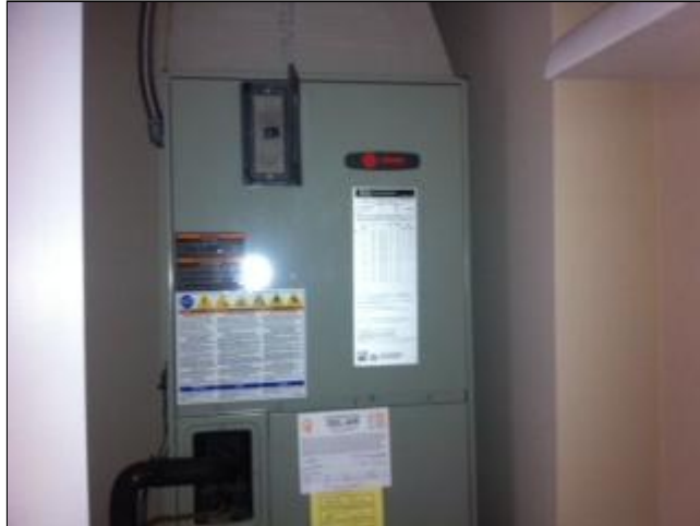
8.8 Picture 1 air handler
